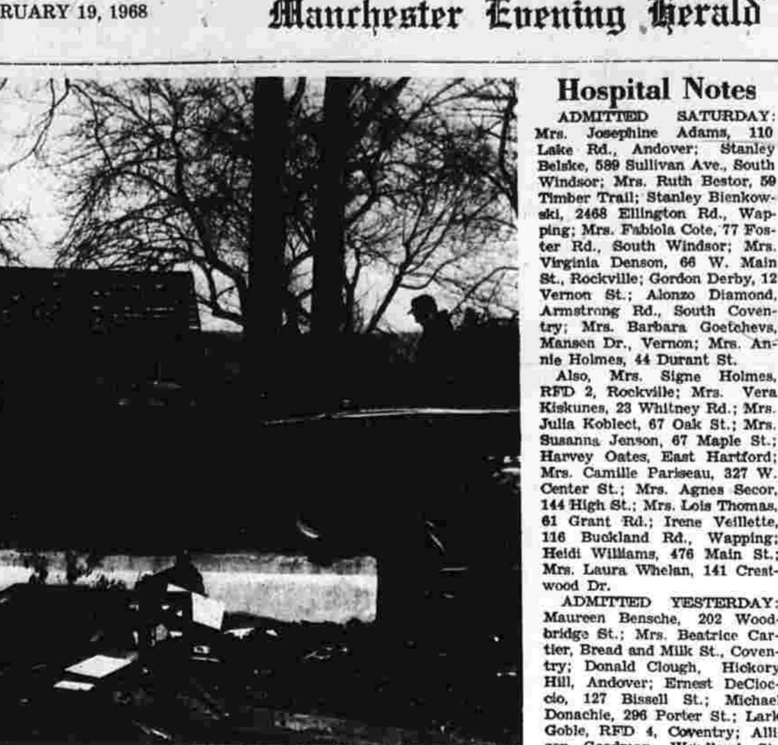
This flatbed truck stands in the middle of the rubble that yesterday was a large garage at the back of the home of H. Calvin Hutchinson at 1071 E. Middle Tpk.
